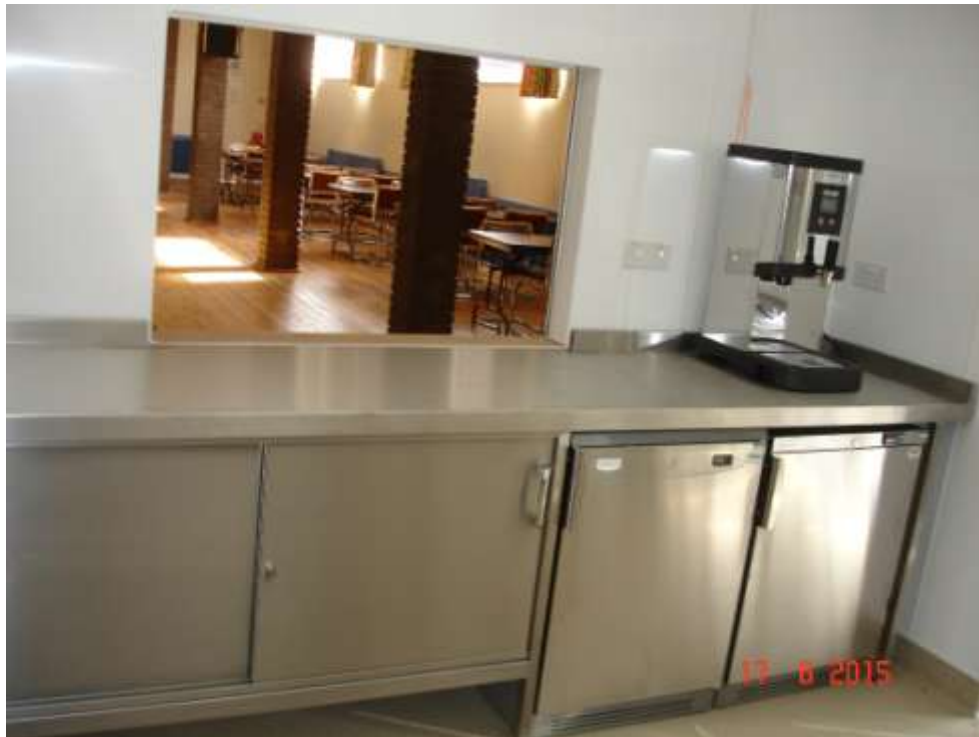
Kitchen Serving Hatch, fridge, freezer and water boiler
